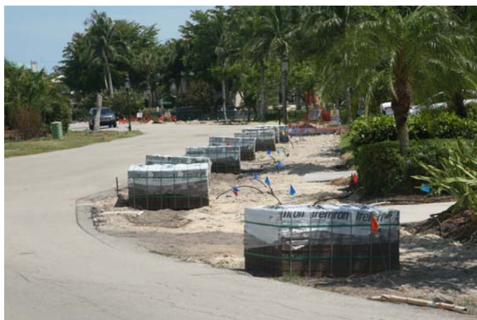
According to Kenneth R Edelbrock from the BBMA "The work on the trees and the sidewalk is moving very well. They started on both ends for the sidewalk and have all of the trees removed. Currently, work consists of installing irrigation lines and then tree planting will begin."
